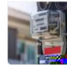
Centralized electricity meter reading
